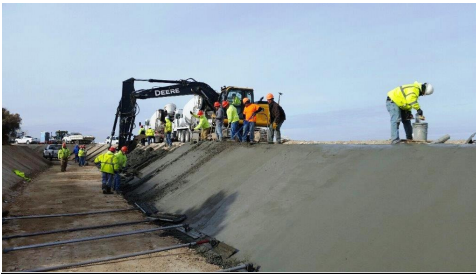
Last November NMID workers lined some 1,300 feet of the Ridenbaugh Canal west of Linder Road with 920 cubic yards of concrete. NMID Photo
