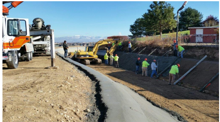
Nampa & Meridian workers install concrete lining on the banks of the Ridenbaugh Canal near Linder Road in western Ada County. (MNID Photo)
