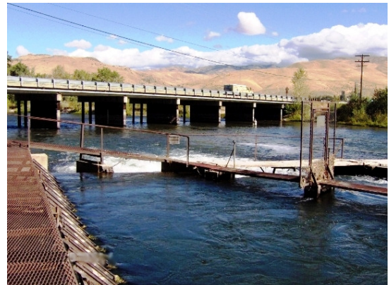
The NMID Boise River diversion near Barber Park will be closed October 11 shutting off the water supply to the District’s historic Ridenbaugh Canal. (NMID Photo)
