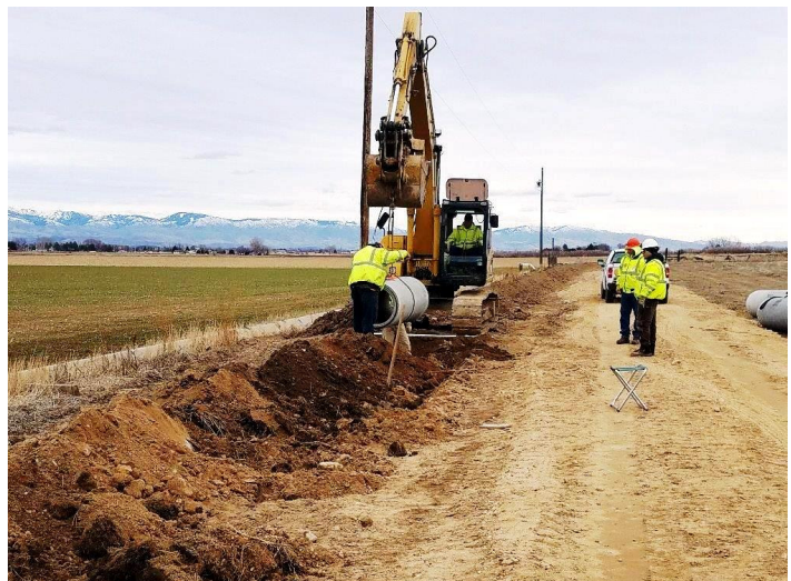
A NMID crew installs 24-inch concrete pipe in farmland to replace more than 1,000 feet of open canal. When the piping project is done irrigation water will be carried underground and the canal filled in with dirt. (NMID Photo)
