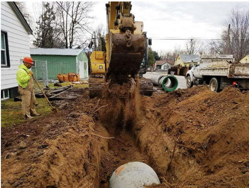
NMID replaced an old metal pipe with 30-inch concrete pipe in a local residential area as part of the District's maintenance projects done while the irrigation delivery system was empty of water. (NMID Photo)
