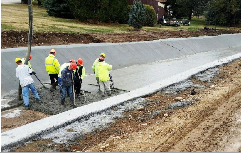
NMID workers pour concrete on the bottom of the Ridenbaugh Canal below Linder Road. More than 1,500 feet of the canal were lined with concrete in the project. (NMID Photo)
